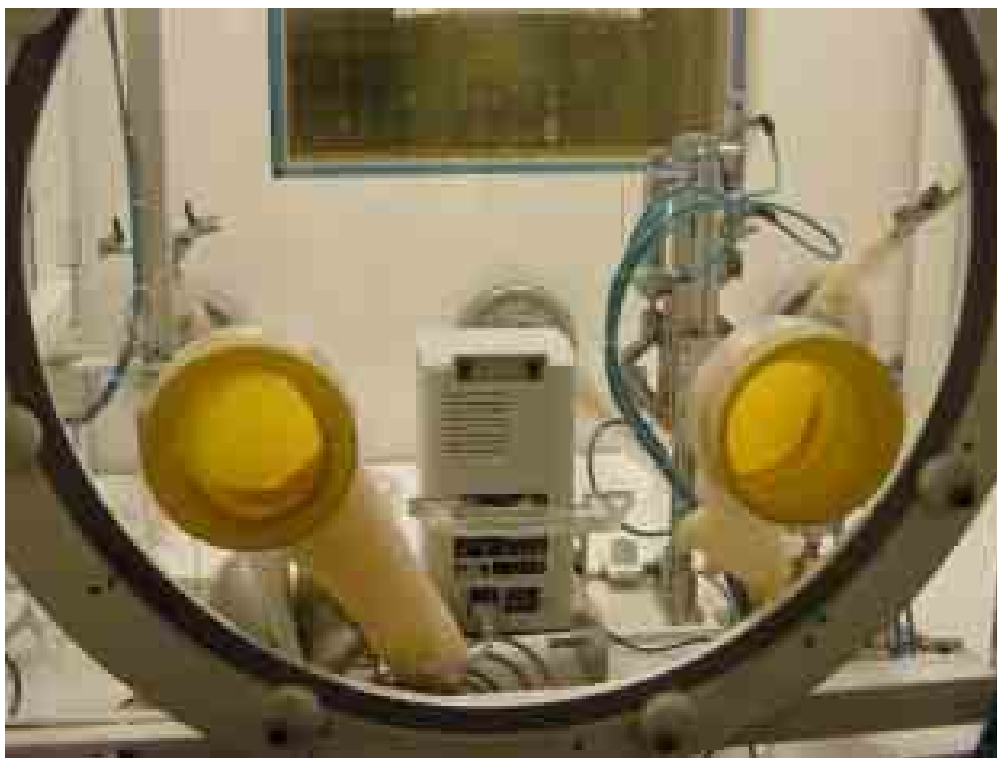
FIG. 6. Rear side of a hot cell with maintenance door (Source: IPEN, Brazil).
