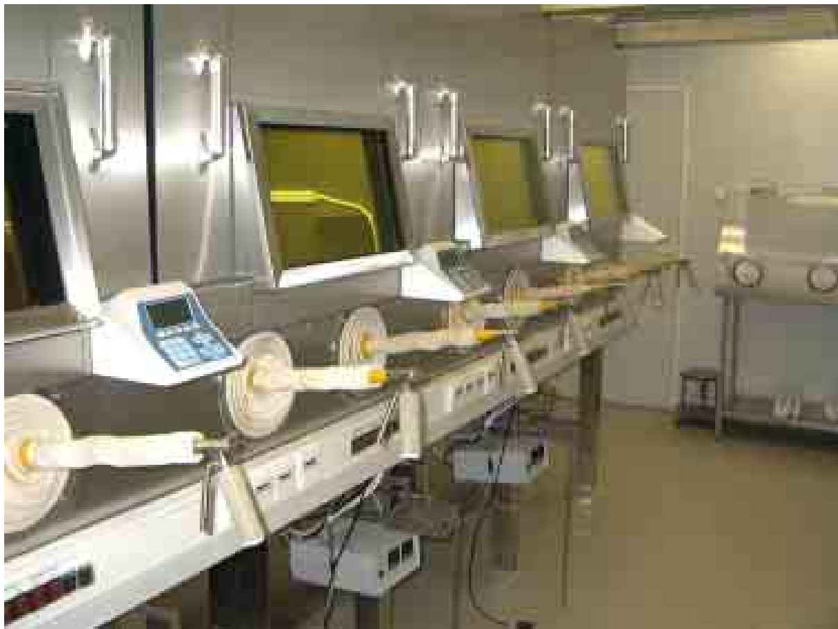
FIG. 14. Hot cells ( -\Delta P ) in clean room ( +\Delta P ) (Source: IZOTOP, Hungary).
