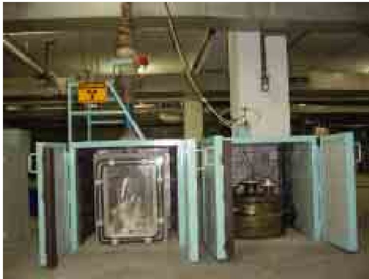
FIG. 5. Solid and liquid radioactive waste disposal equipment (Source: IPEN, Brazil).
