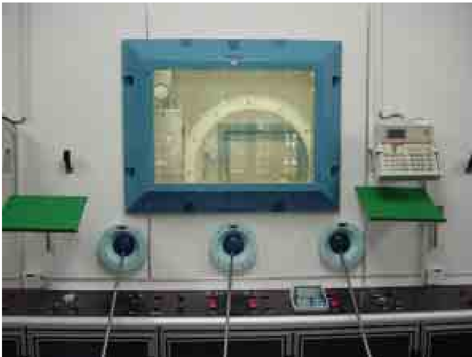
FIG. 4. Front of a hot cell with remote handling tongs (Source: IPEN, Brazil).
