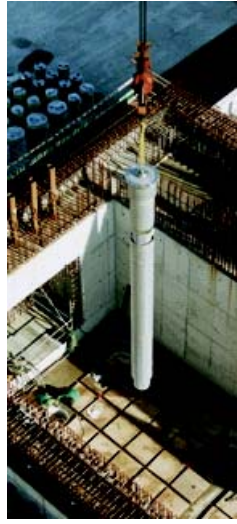
Mounting one of the storage vaults for vitrified HLW in the HABOG
