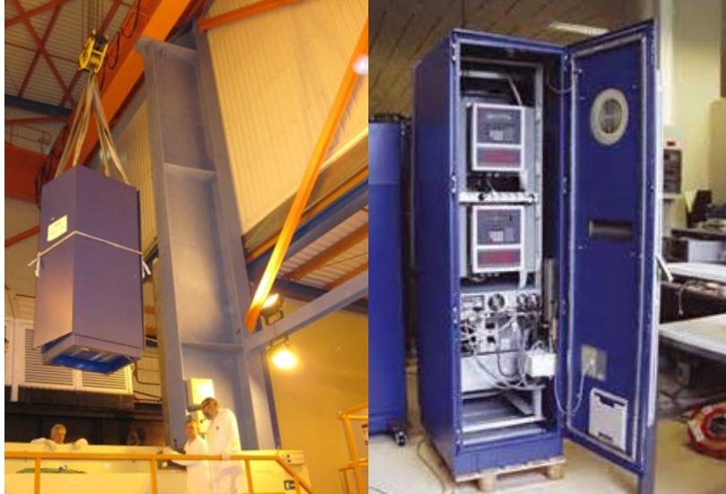
FIG. 8. Operator support to installation of IAEA equipment racks.
