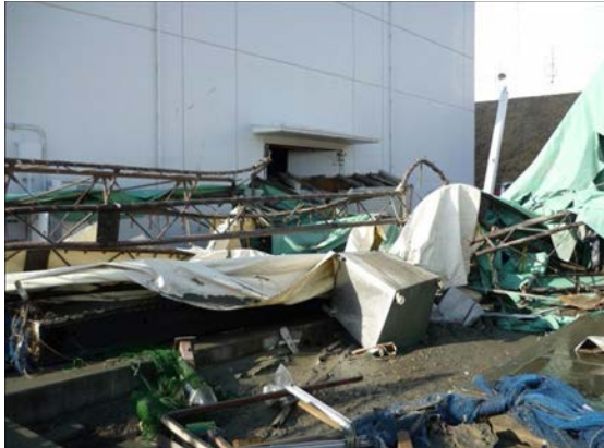
FIG. 34. Debris near the heat exchanger building of Fukushima Daini nuclear power plant, Unit 3. Reproduced courtesy of Tokyo Electric Power Company [64].
