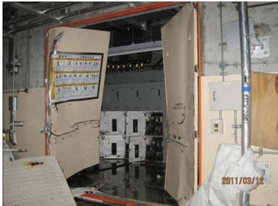
FIG. 32. Damaged door of the heat exchanger buildings. Reproduced courtesy of Tokyo Electric Power Company [64].
