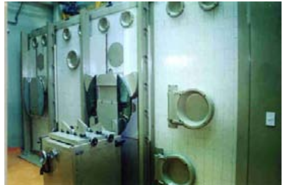
Fig. 8 – LFR hot-cells line, rear view (Controlled Area).
