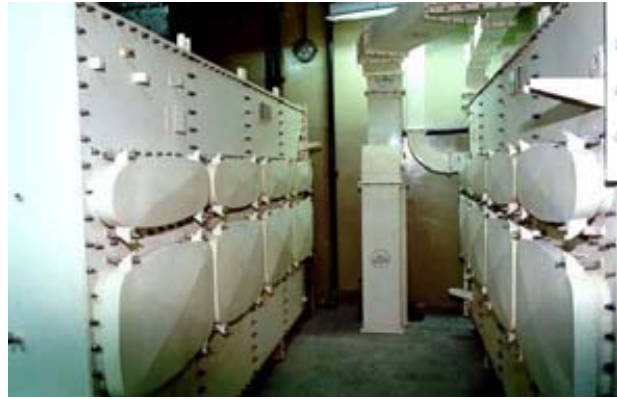
Fig. 3 – LFR Filtration Room.
