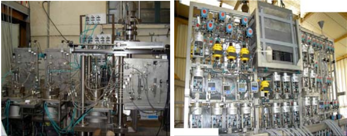
Figures 7 & 8 present the corrosion loop with the autoclaves (now inside the hot cell) and its regulation system.
