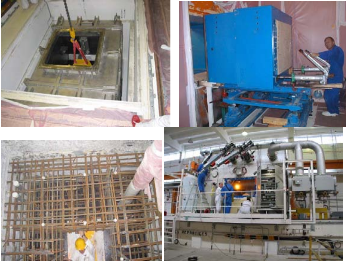
Figures 12 to 15: a stainless steel confinement box is inserted inside a LECA hot cell (upper left), a new window is put in place (upper right), civil engineering work to reinforce seismic resistance (bottom left), a new mobile hot cell has been constructed on the roofs of the concrete shielded line to improve confinement when opening cell roof (bottom right).
