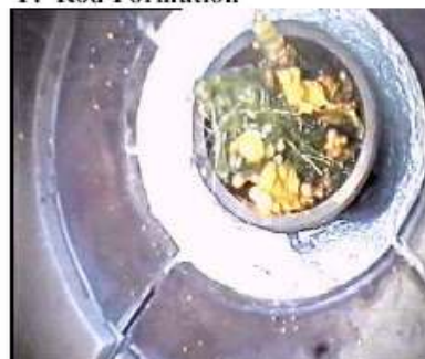
H. Susceptor choking during Sulphate draining (yellow phase mainly consists of sodium sulphate)
