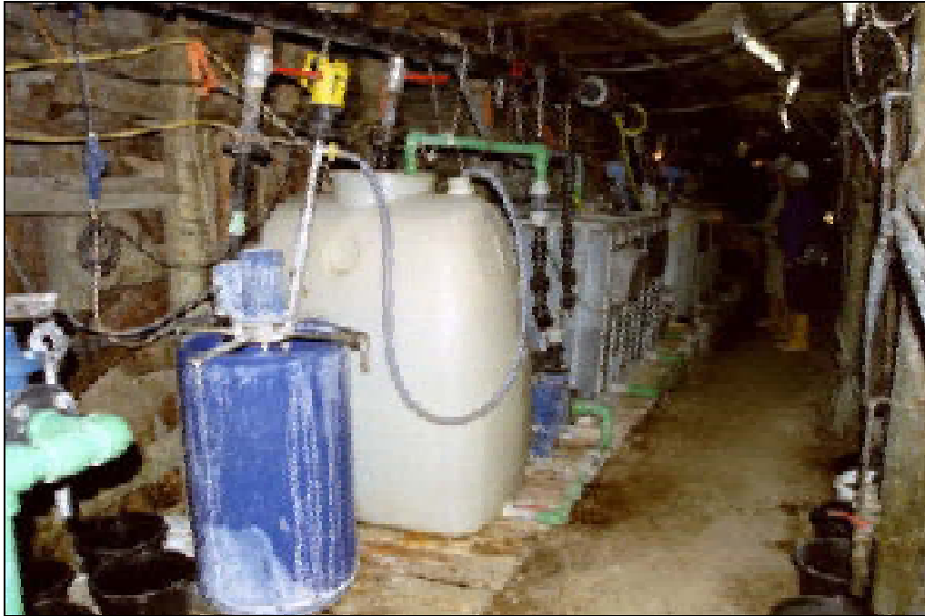
Fig. VI-49. View of the grout plant used for the preparation of the BaSO 4 forming solution.
