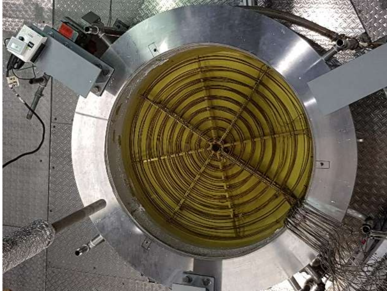
FIG. 6. Top-view of the LIVE-CC facility filled with molten salt and heated by several layers of resistors.
