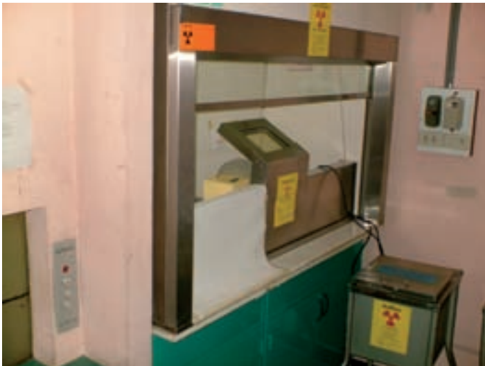
FIG. 5. Typical fume hood.
