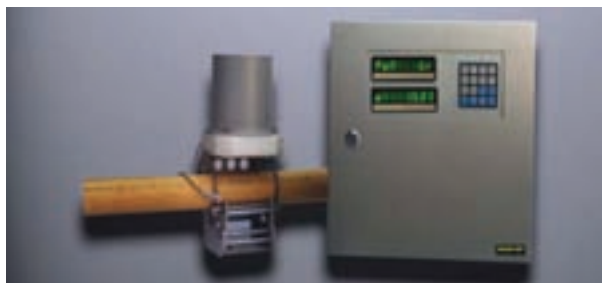
FIG. 70. Typical ^{241}\text{Am} transmission gauge installed on a section of pipe.
