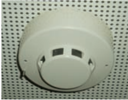
FIG. 97. Typical smoke detector (front view).
