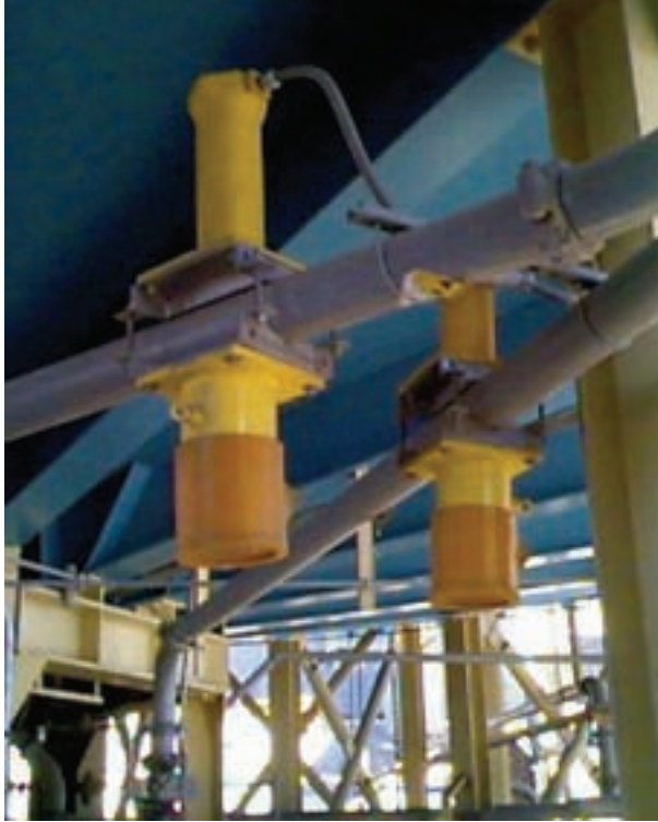
FIG. 66. Pipeline density gauges in position.
