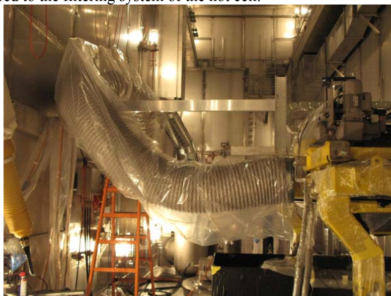
FIG. 3: Suction system in the hot cell, to prevent a spread of contamination.
