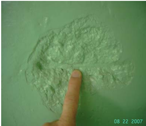
Fig. 5. Showing reinforcement (painted over) that had corroded and fractured concrete
