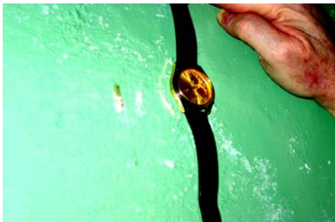
Fig. 7. Showing white deposits formed by water
