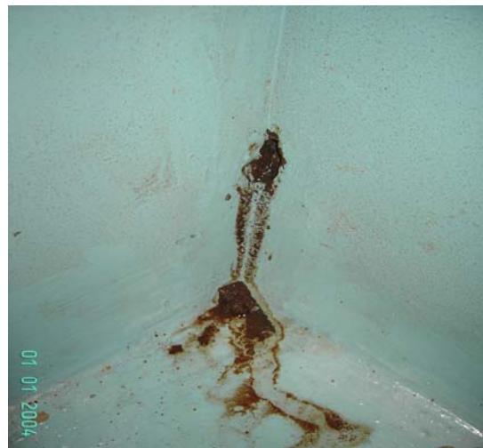
Fig. 9. Showing water and 'mud' seeping from the reactor block wall.
