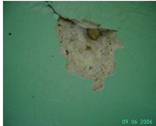
Fig. 6. Showing a clay nodule that had expanded and fractured the concrete
