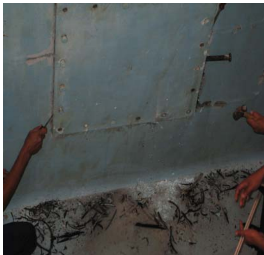
Fig. 8. Showing water leaking from the thermal column
