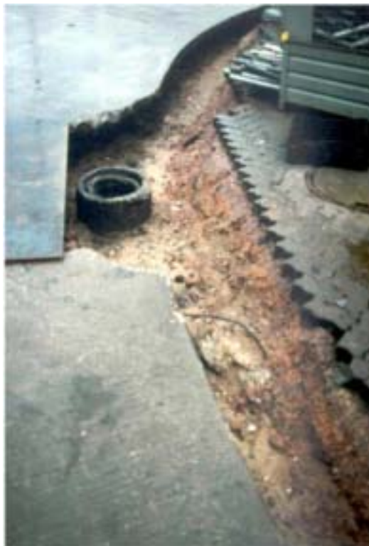
FIG. 14. Control measurements of drains at HDR.
