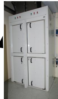
Filter tower for retaining radio-iodine
