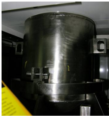
Docking of container below hot cell-1 of Mo-99 Facility
