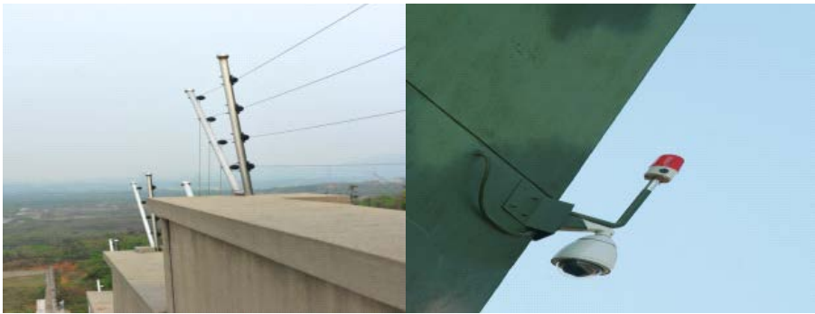
FIG. 4. Electronic perimeter fence and infrared detector.
