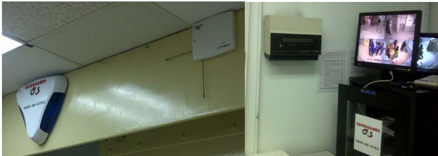
FIG. 4. Intrusion alarm system and monitoring devices installed at a radiotherapy department.
