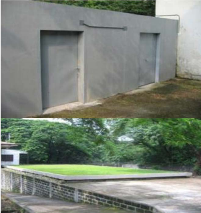
FIG. 1. PNRI interim storage facilities.
