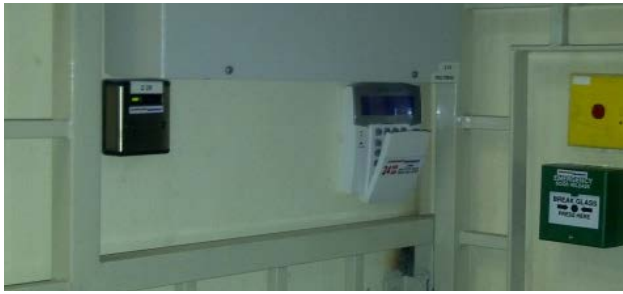
FIG. 3. Proximity card reader installed for access control.
