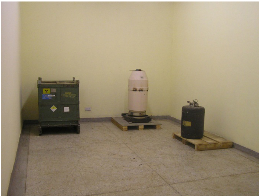
FIG. 64. Storage of DSRs on the floor in the intrusion resistant room.
