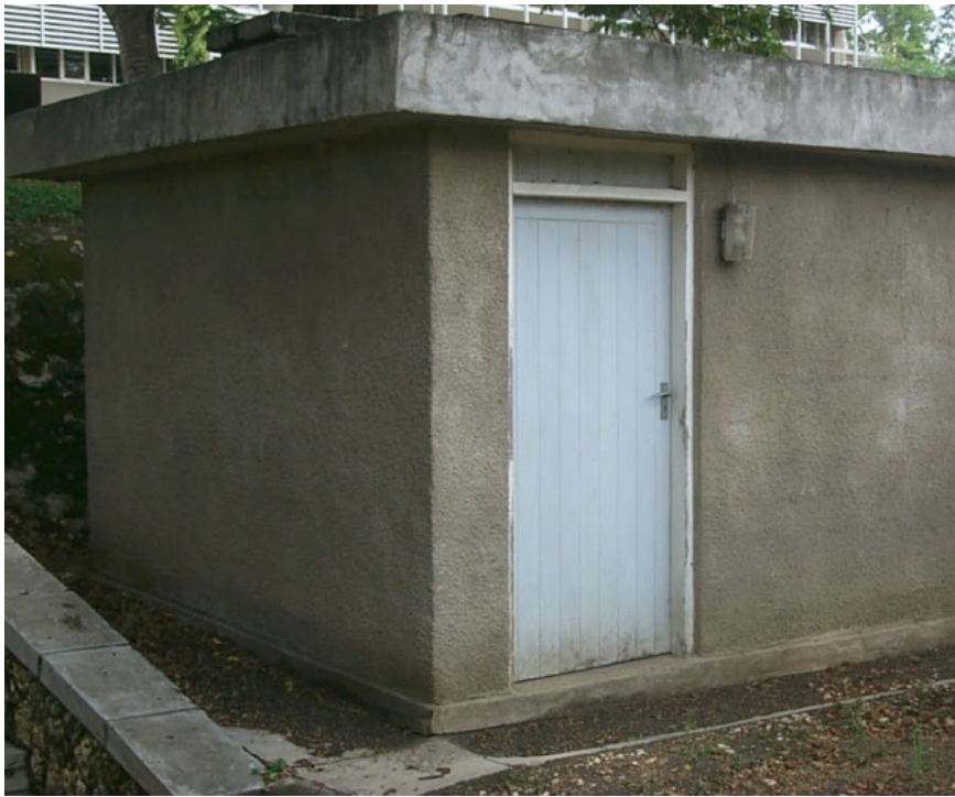
FIG. 72. A storage building without a warning sign or label.
