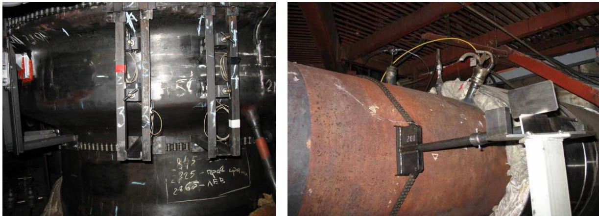
FIG. 41. Mounting of the acoustic emission, ultrasonic and displacement sensors.
