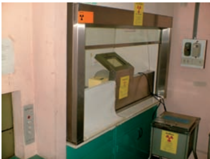
FIG. 5. Typical fume hood.
