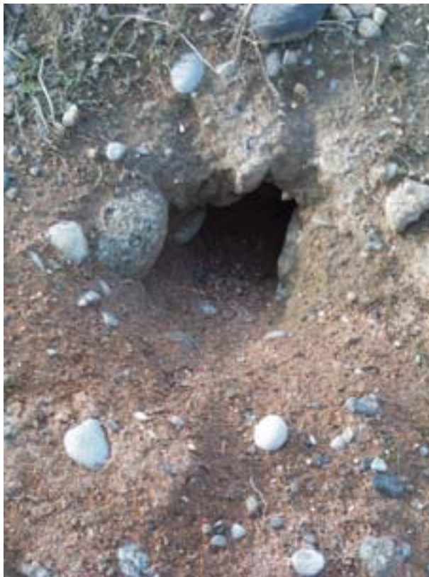
FIG. 14. Hole in an embankment made by a burrowing animal.
