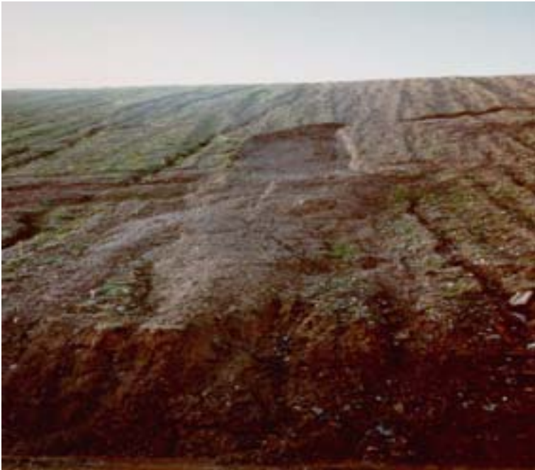
FIG. 12. Cracks and sliding of a pile cover
