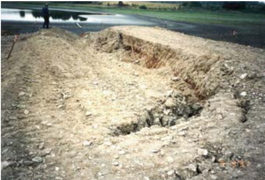
FIG. 15. Differential settling of a pond cover.
