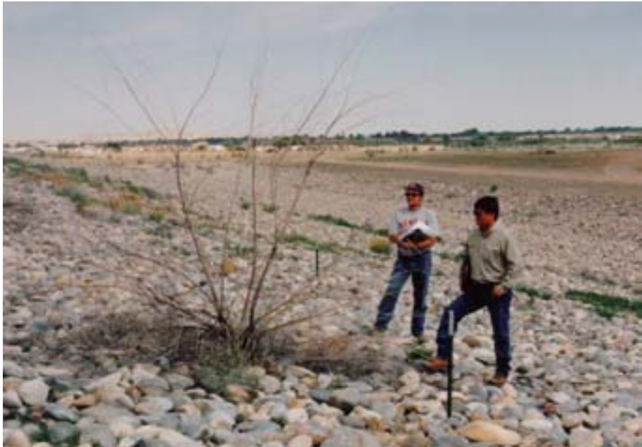
FIG. 13. Shrubs growing on a covered embankment.
