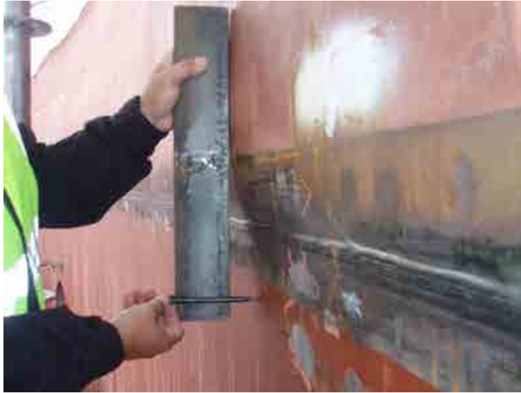
FIG. 22. Problems revealed by weld inspections of containment steel liner during Olkiluoto 3 construction (courtesy of STUK).
