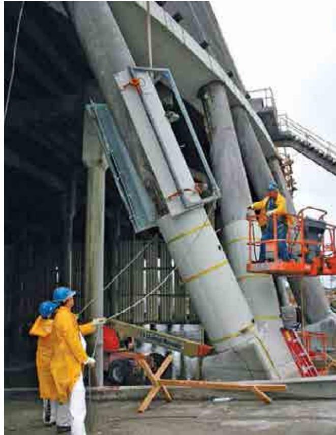
FIG. 162. Cathodic protection system being installed as part of cooling tower concrete repair [555].
