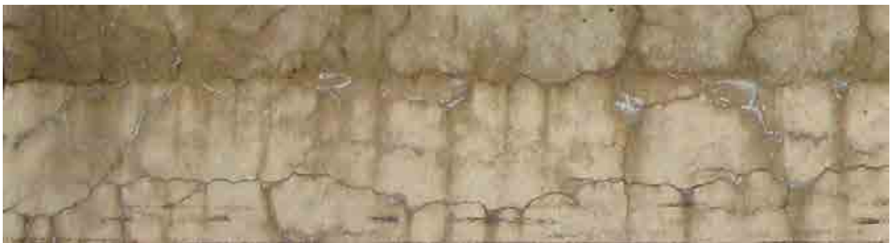
FIG. 38. Example of cracking and gel resulting from ASRs in concrete (courtesy of CTLGROUP) [139].
