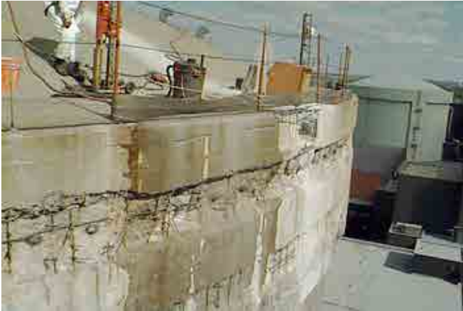
(a) Before repair, 1999.
