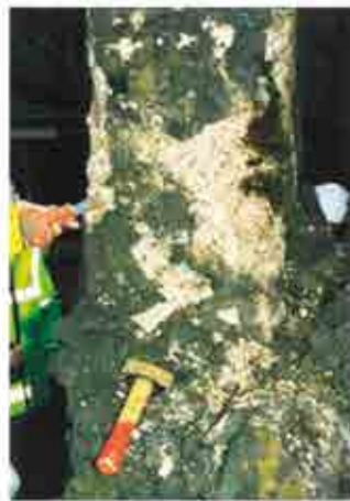
Subsurface concrete pier affected by thaumasite sulphate attack.
