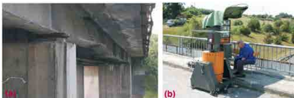
FIG. 70. Application of modal analysis to a damaged bridge girder: (a) view of damaged main girder; (b) electrodynamic exciter placement on a bridge [367].
