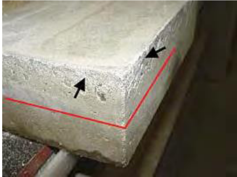
FIG. 26. Concrete slab experiencing deterioration due to salt crystallization; arrows indicate concrete surface deterioration and lines indicate the level of solution in wetting cycle [90].
