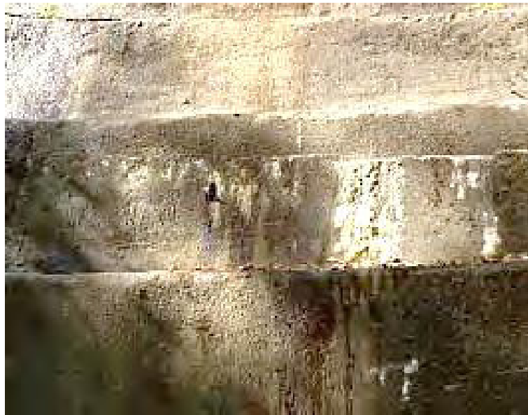
FIG. 31. Efflorescence in a water retaining structure [123].
