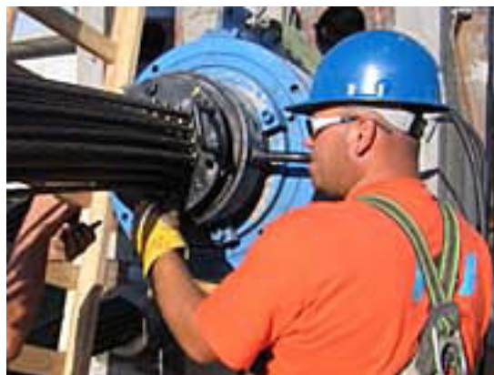
FIG. 19. Steel tendons (courtesy of Oak Ridge National Laboratory).
