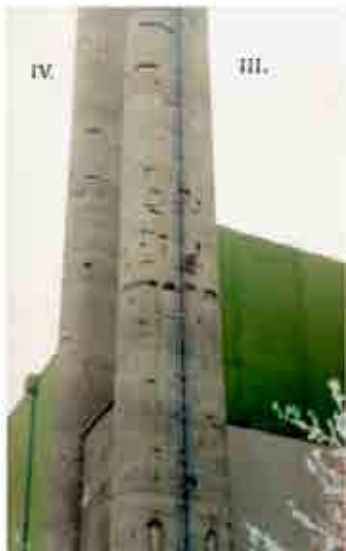
FIG. 201. Conditions before repair.
