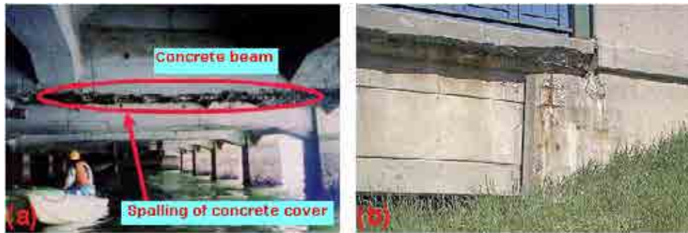
FIG. 45. Corrosion of reinforced concrete. (a) Seawater structure; (b) bridge structure on highway 401 in Ontario, Canada (adapted from Refs [160] and [161], respectively).
