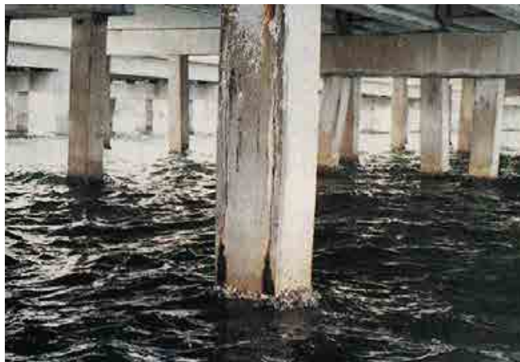
FIG. 40. Seawater damage to concrete [146].
