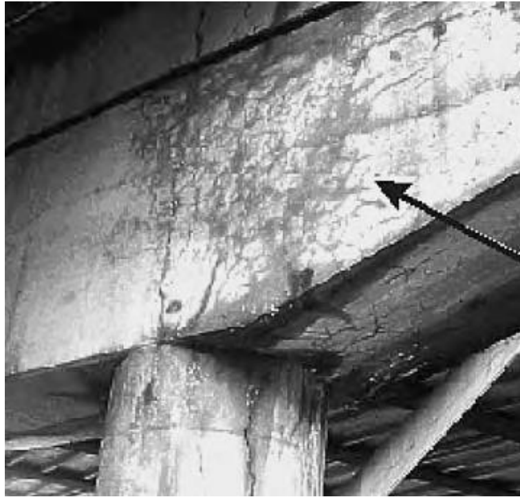
FIG. 35. Cracking damage in a concrete structure due to DEF [131].
