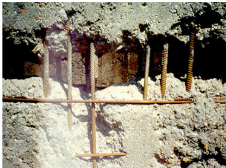
FIG. 202. Conditions before repair.
