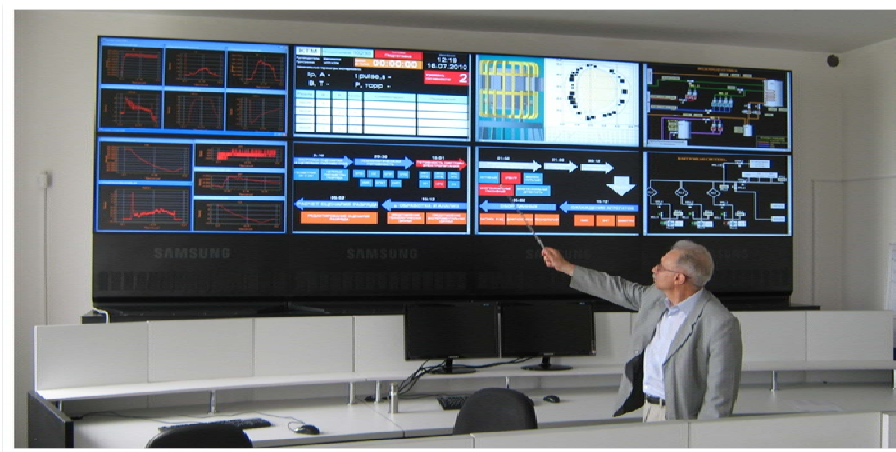
FIG. 2. KTM control panel
