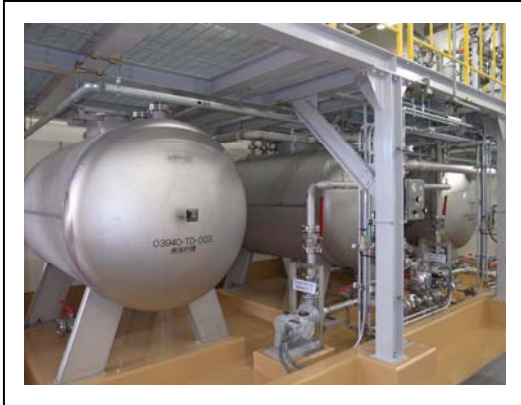
Fig. 2 Installation of tritium waste water processing system.
